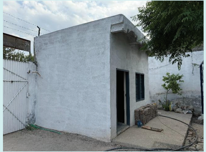
Fig-29: new room constructed without earthquake resistant elements.
