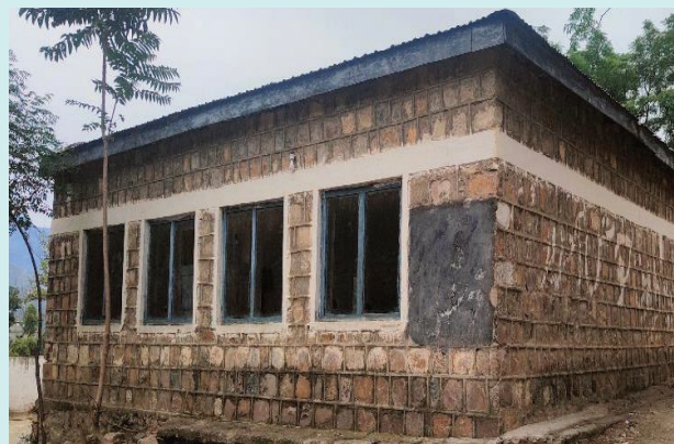
Fig-21: A school building with a lintel band, may be unreinforced and only architectural.
