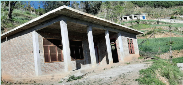
A post-2007 school building with RC frame at the front but lacking reinforcement.
