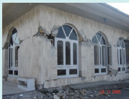
h. Rocking and crushing of piers
