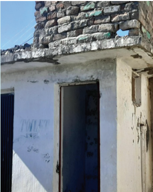
Fig-18: Parapet falling hazard
