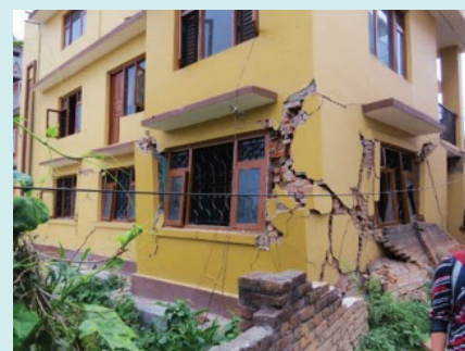
i. Crushing of masonry pier
