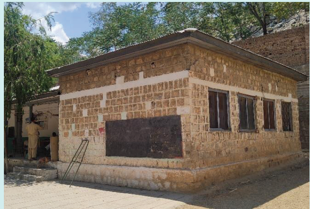
Fig-4b. Stone masonry building apparently with a discontinued reinforced concrete
