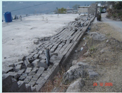
b. Collapse of parapet during the Kashmir earthquake
