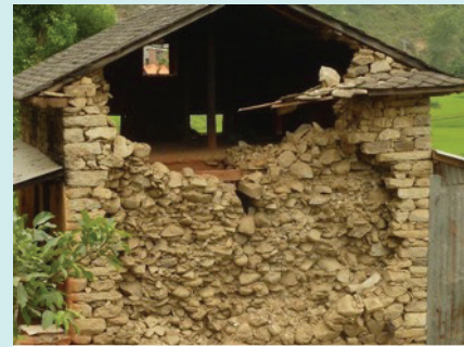
c. A stone masonry building with delaminated wall. Also note collapse of gable
