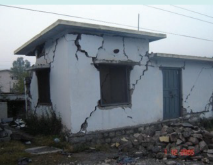
g. Diagonal shear cracks
