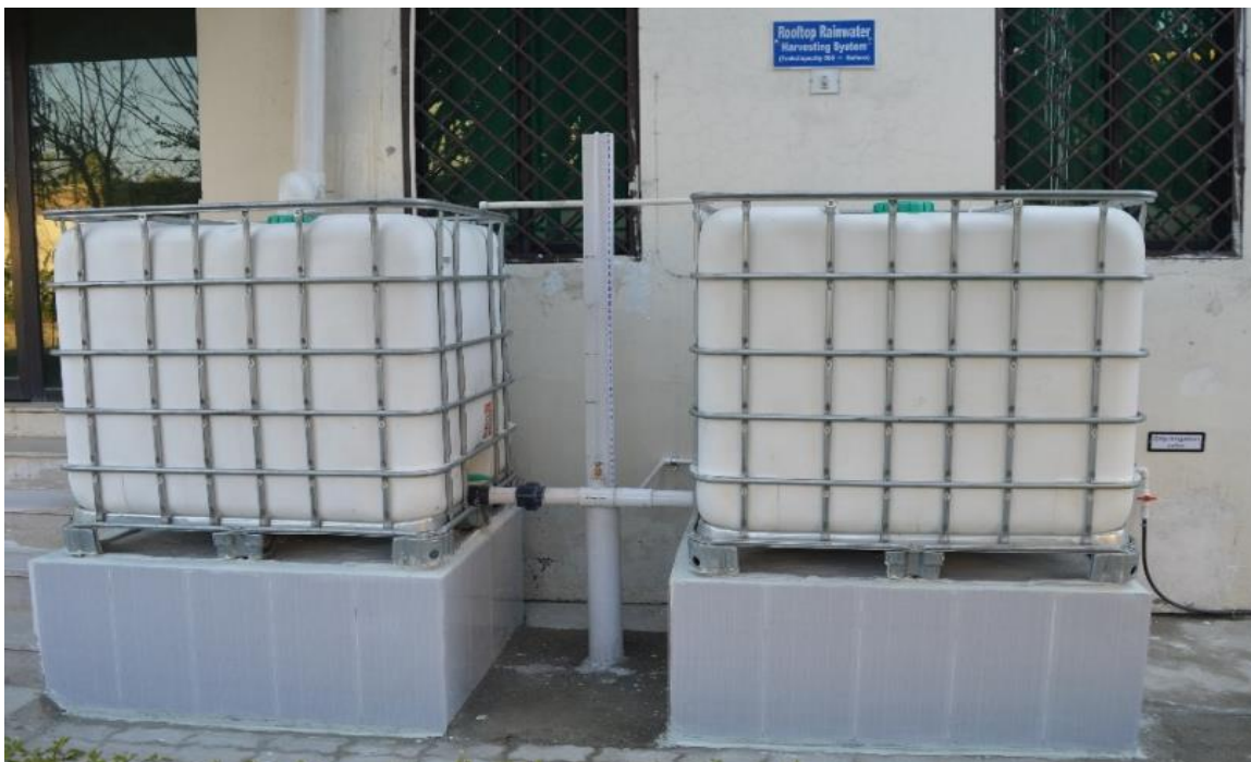
Figure 7: Rooftop Rainwater Harvesting Storage Tanks Installed at PCRWR
