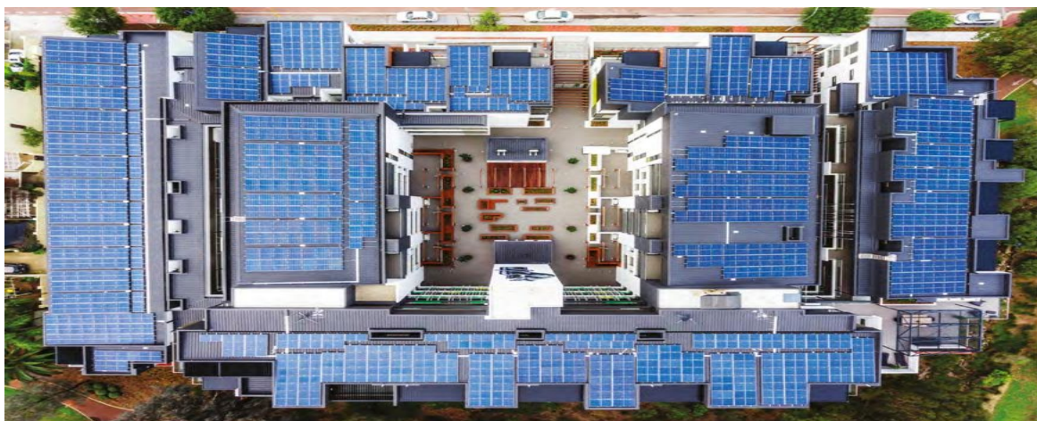
Apartments utilizing roof with installation of photovoltaic arrays to supplement power consumption of dwelling units
