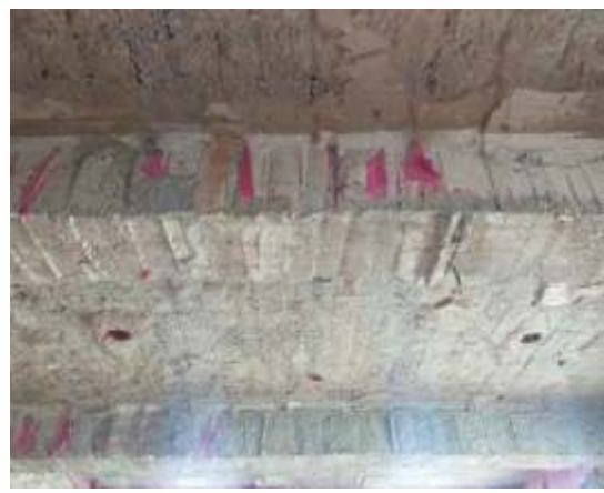
Existing poor construction mortar and improper concrete cover exposed
