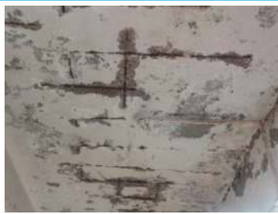
Steel exposed due to bond failure and seepage
