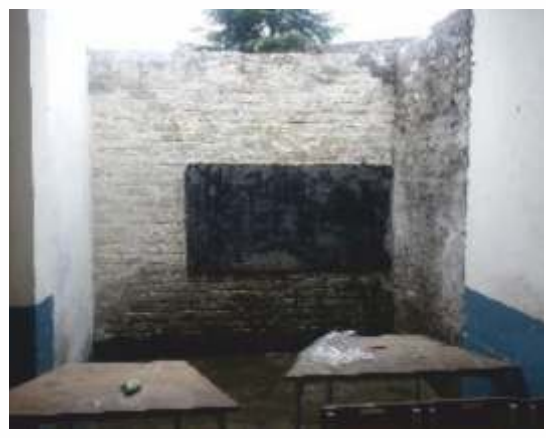
Open classroom with damaged walls
