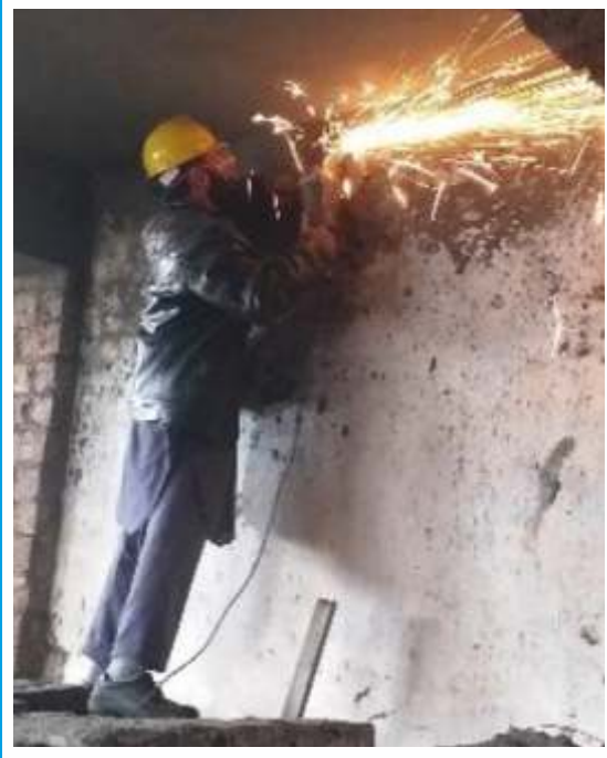
Cutting of existing oxidized steel of beam to reduce the rust impact on inner
