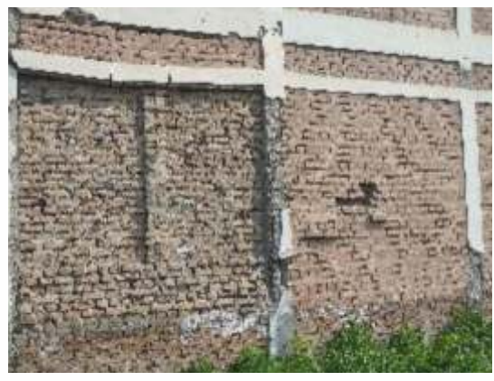
Buckling of walls and column, sag in beam
