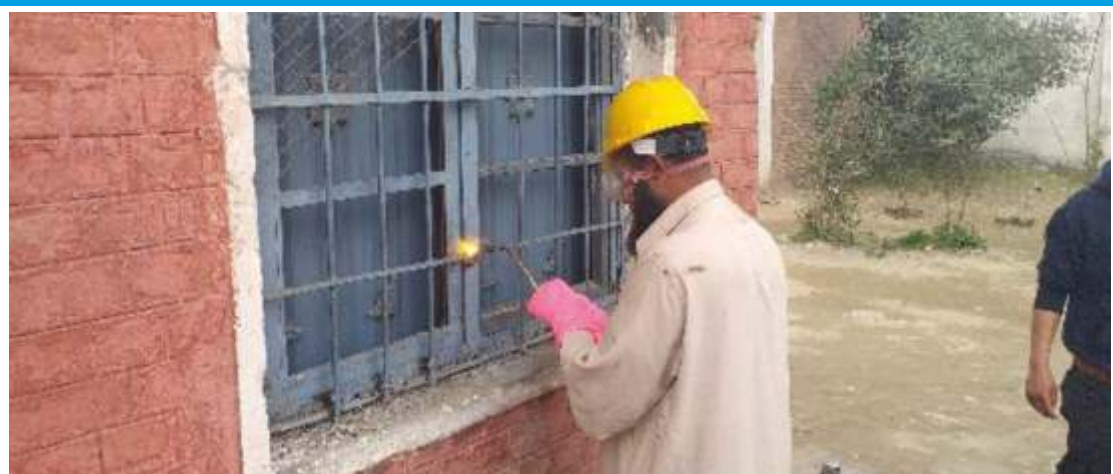
Repairing of windows by apply new mesh using gas welding for heavy-duty joints
