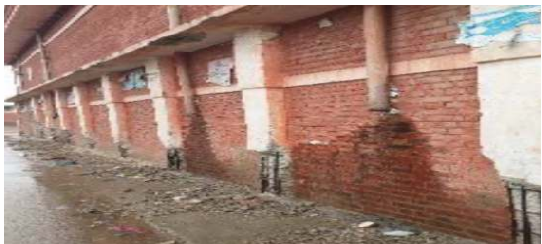
Dismantling of weak/damaged parts of RCC columns and cleaning of rust from steel
