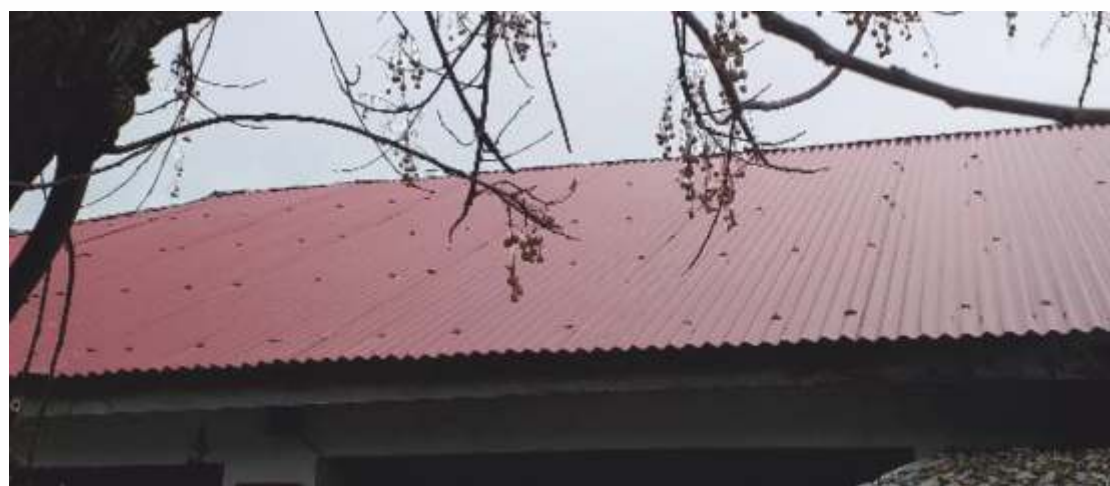
Fixing of new CGI sheets over whole roof by in order to avoid leakage during rain
