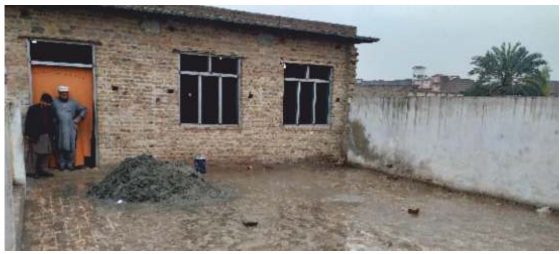
Brick flooring causes seepage and weaken the slab of ground floor
