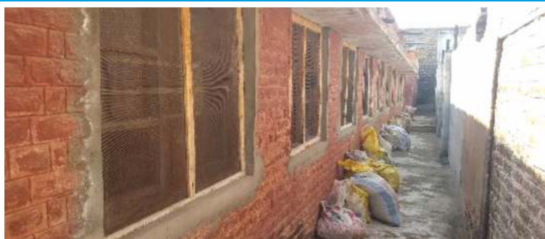
Repairing of windows by apply new mesh using gas welding for heavy-duty joints
