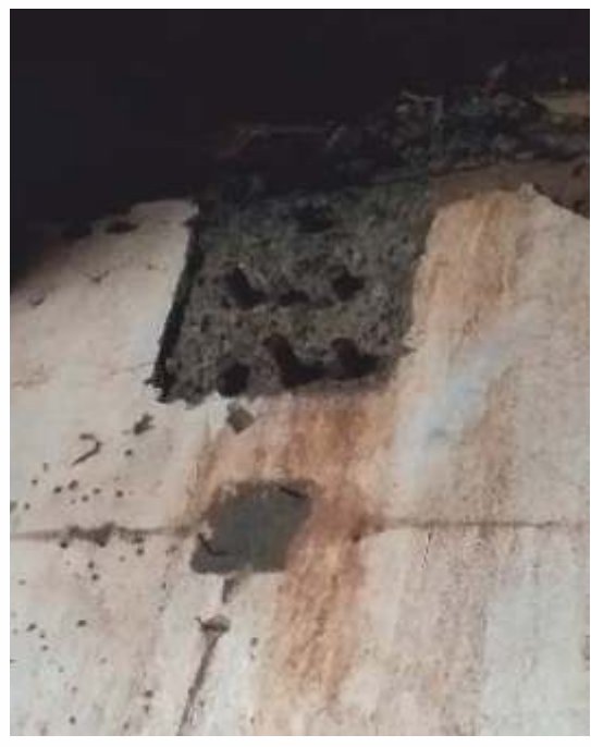
Steel left outside the beam due to previous poor construction reinforcement
