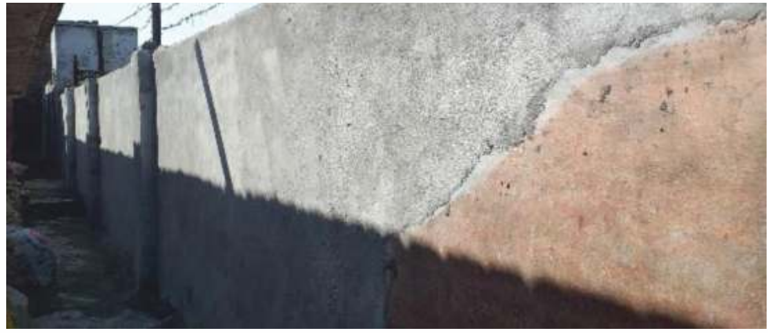
Retrofitting of boundary wall next to river can be a hazard in flood
