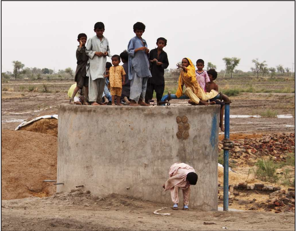
Construction of water supply system on village common land in Jacobabad, Sindh, Pakistan
